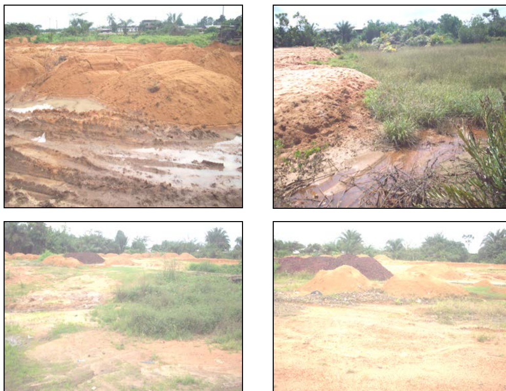
Figure no. 11 The reclamation process around Bikoko by the use of earth and scoriaceous deposits
